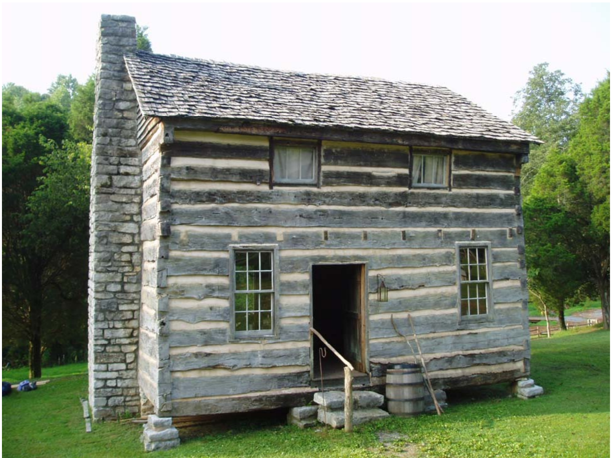
Figure 2. The two-story Walker Springs cabin sits near the Governor John Sevier cabin, but was relocated to the Marble Springs Historic Site in 1988. View is of the north side. Note the differences in log sizes and their state of preservation in this cabin with logs in the Gov. John Sevier cabin (Figure 1).
