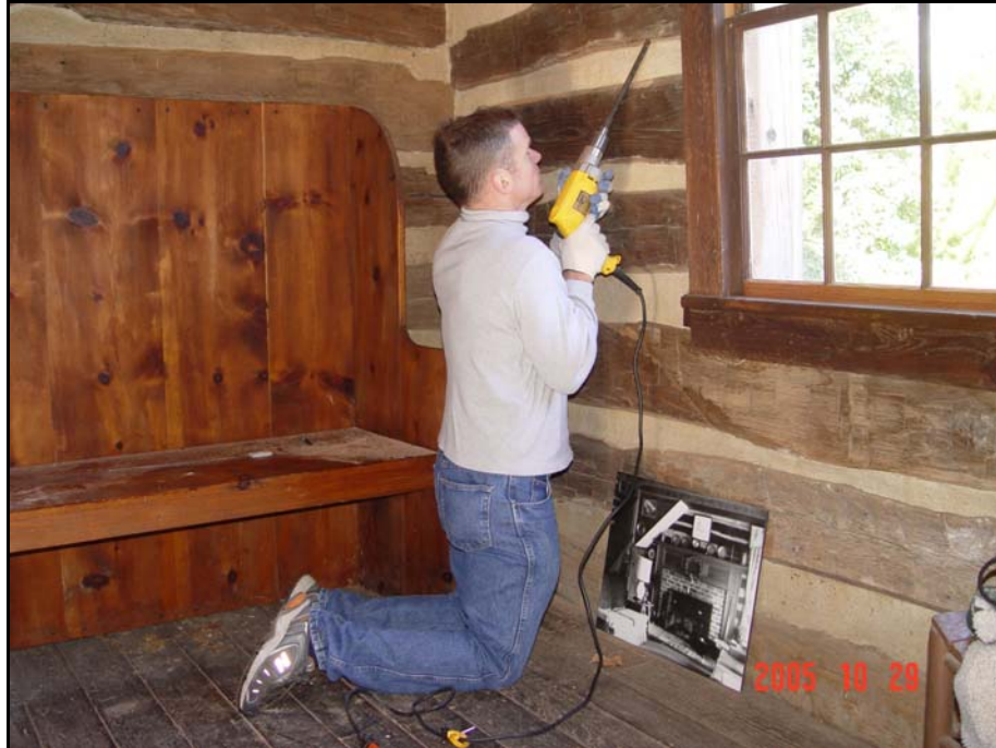
Figure 2. Joe Henderson shown extracting a core from the rounded portion of a log in the Hoskins House with a hollow tubular drill bit.
